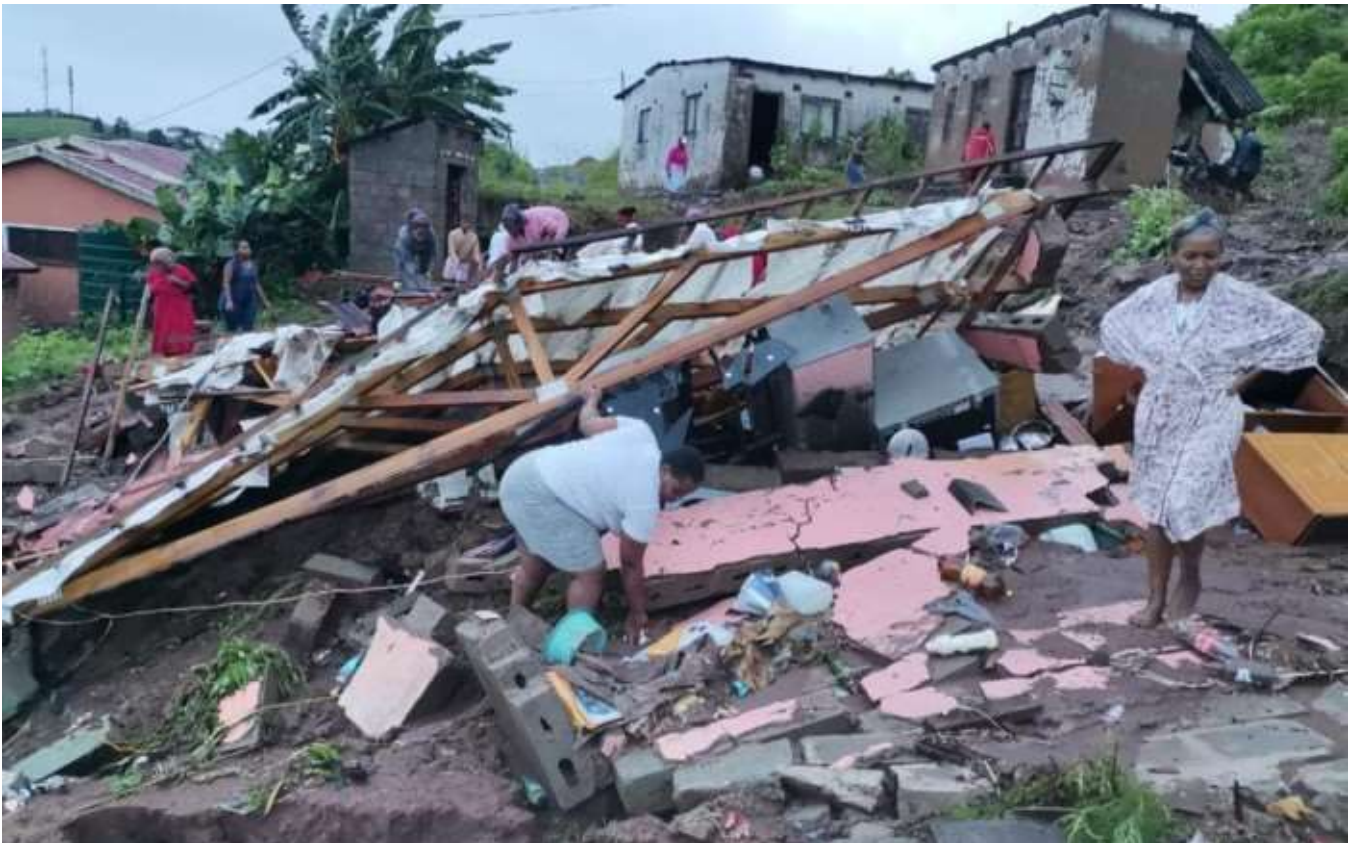
Catastrophic flood damage in KwaZulu Natal
